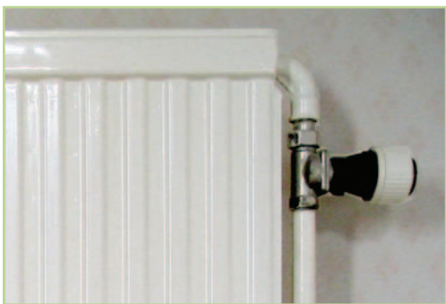
Radiator valve at a height of 800 mm
